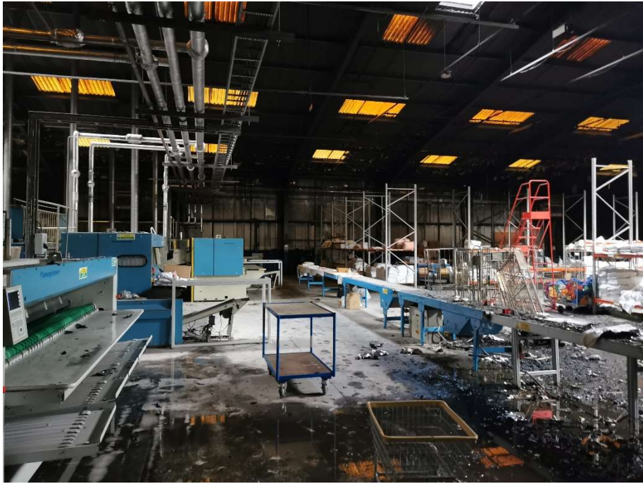
21. General overview of fire damage in Unit 2a.
