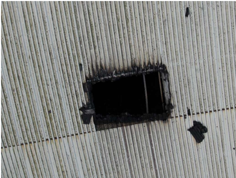
8. Fire damaged caused to the roof.
