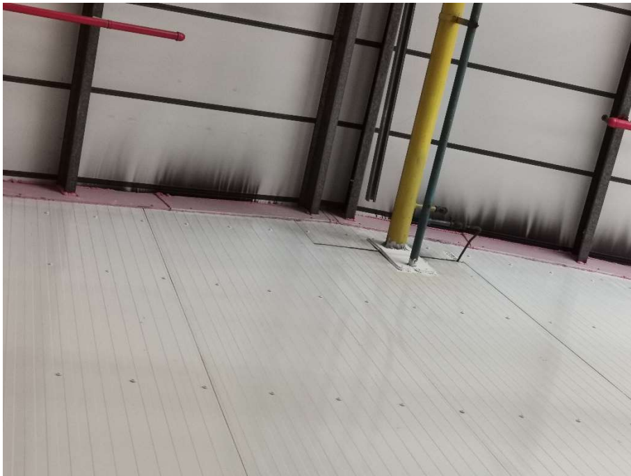
26. Smoke damage to the underside of the roof to Unit 1 at the party wall junction with Unit 2a.
