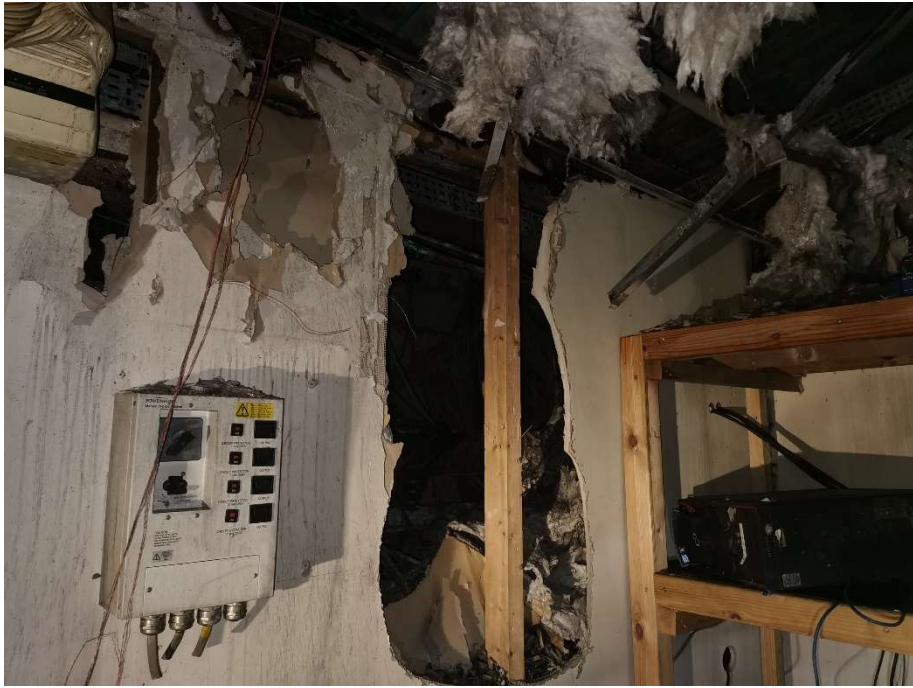
11. Server room at first floor level within Unit 2b.
