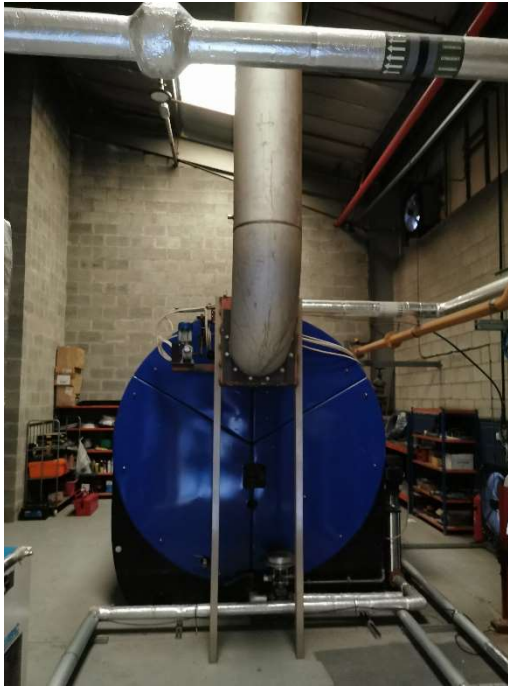
25. Overview of boiler located in plant room to Unit 2a.
