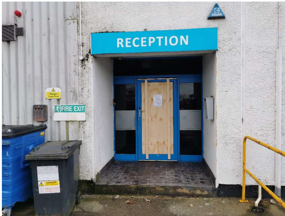
3. Damaged door to Unit 2b.
