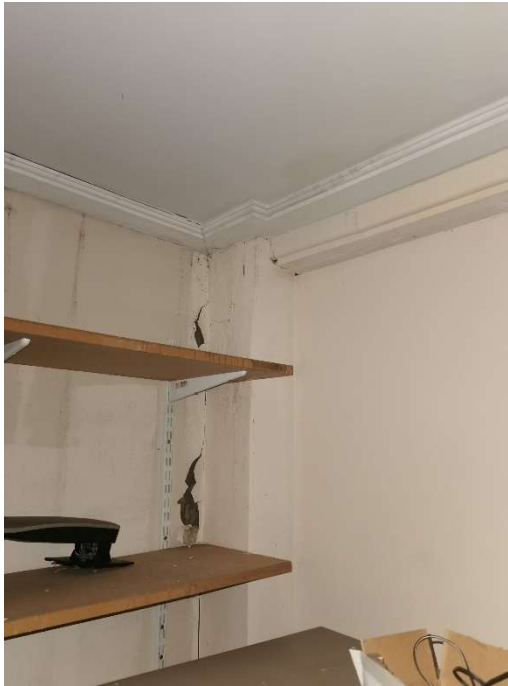
15. Water and smoke damage to Unit 2b at ground floor level.
