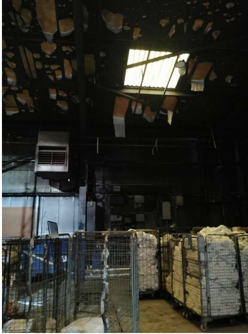
19. General overview of fire damage in Unit 2a.
