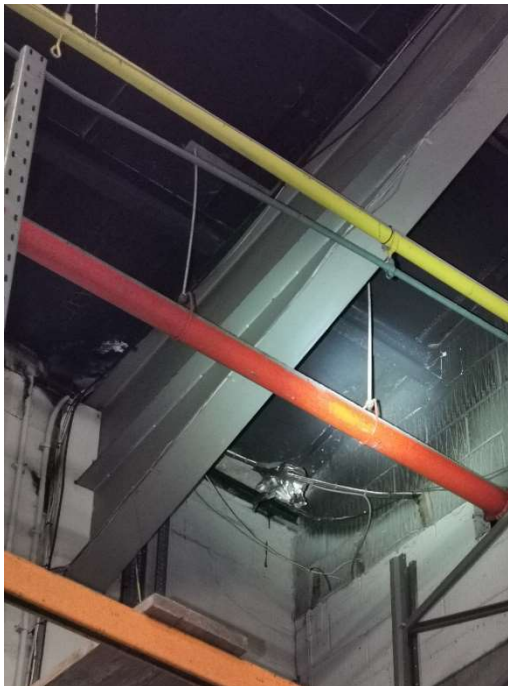
14. Smoke damage to roof in Unit 3.
