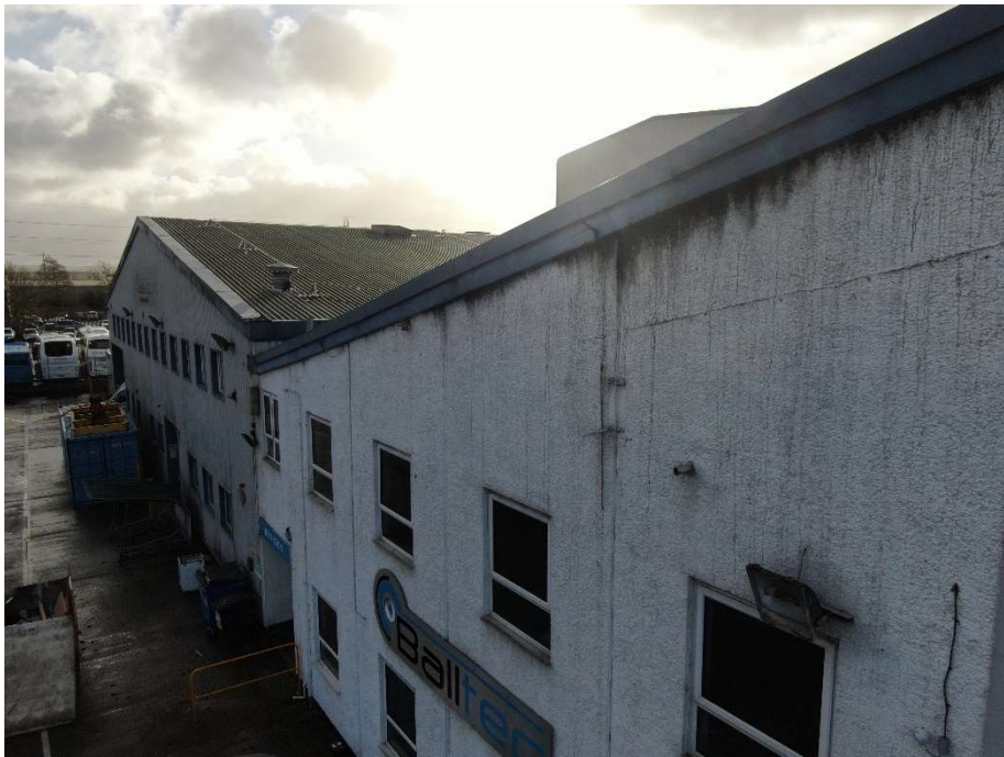
6. Smoke damage below the verge trim.
