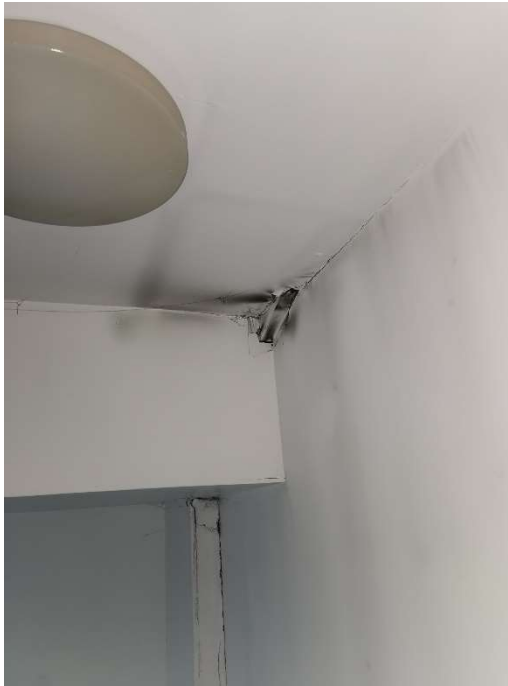
23. Smoke damage to staircase leading up to meeting room in Unit 2a.
