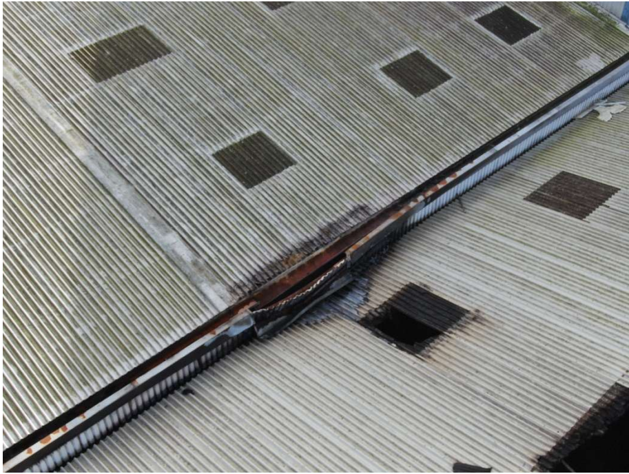
5. Overview of roof showing damage caused by the fire.
