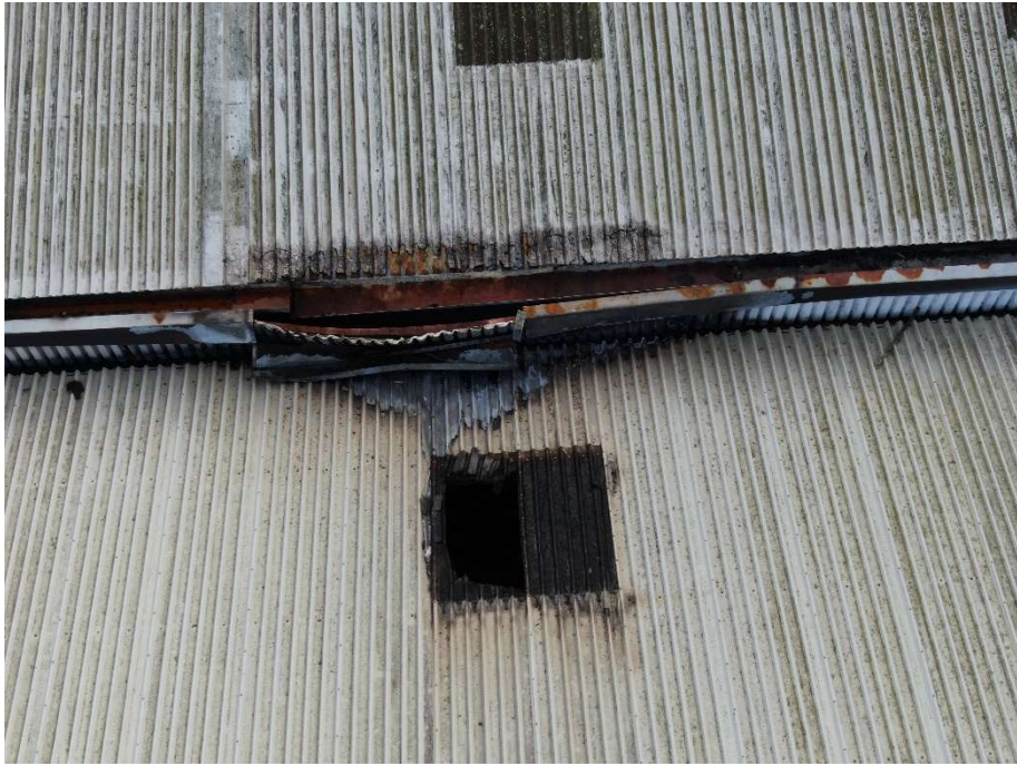
9. Fire damaged caused to the roof.
